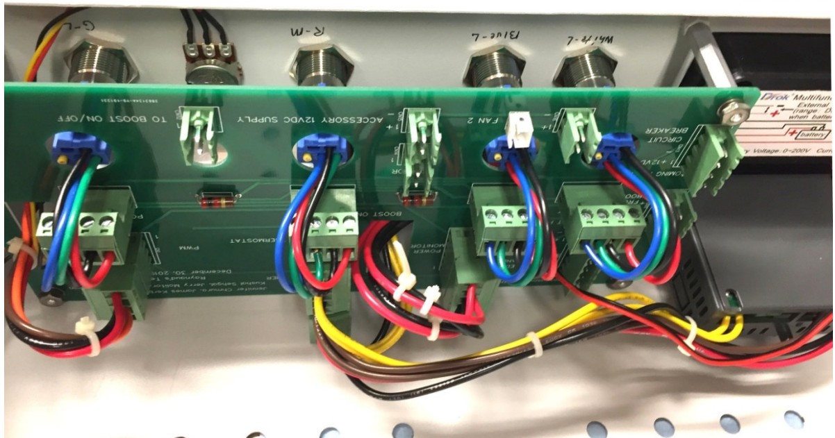
Inverted Top Section, PCB Placement behind Control Panel Cluster
